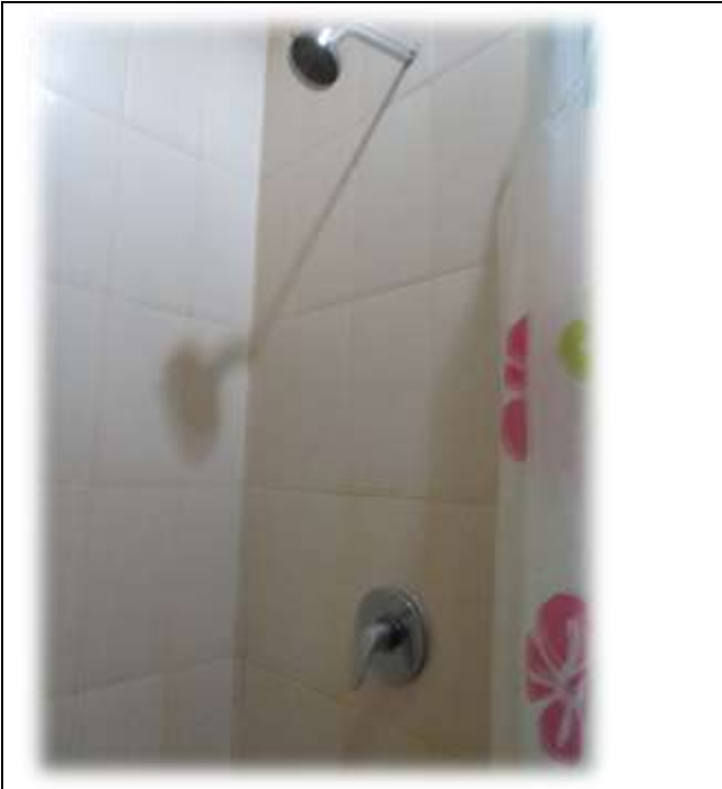
Figure 01: Water efficient appliances are applied in the use of bath shower in UNS INN, LPPM Office, Rectorat Office, PPLH Office and Postgraduate Office.
