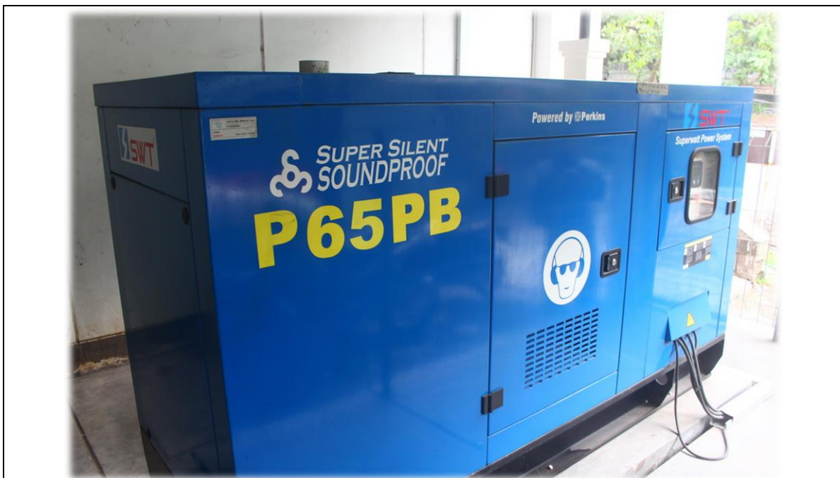
Figure 01. The use of environmental-friendly Genset in UNS-hospital
