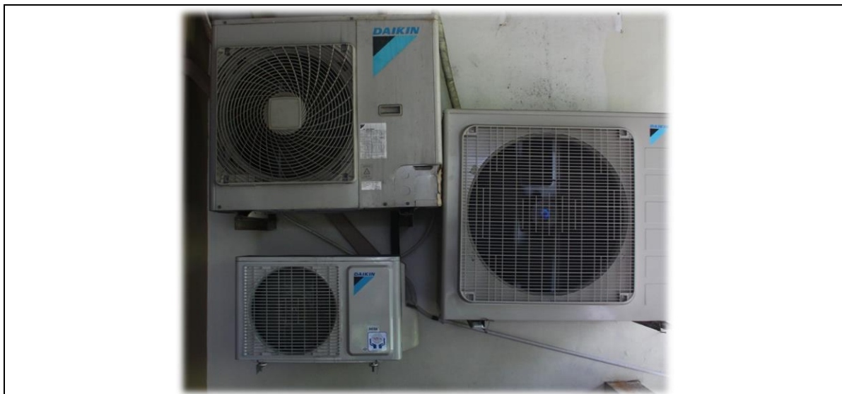
Figure 02. The use of environmental-friendly Air Condition.
